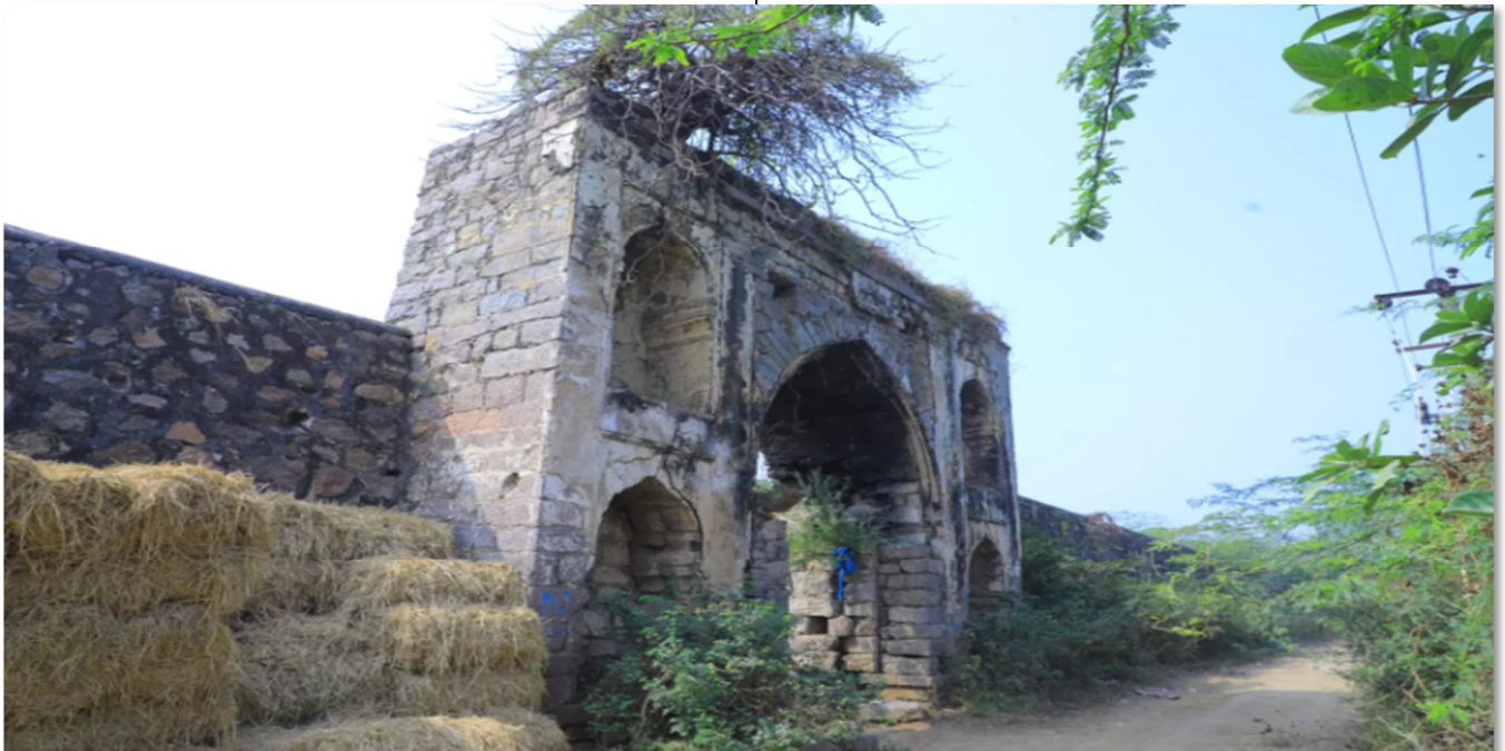
An old gateway and stone walls at Molangur Fort show signs of deterioration.
